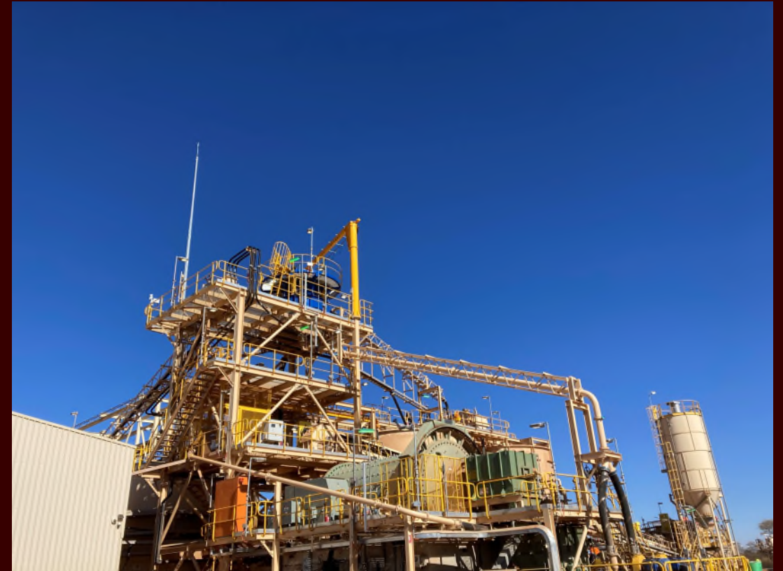
Meeka Metals gold processing facility north of Meekatharra Image: MWDC Bev Brosnan
