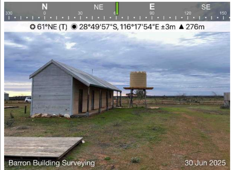
Water storage (150,000lt)
